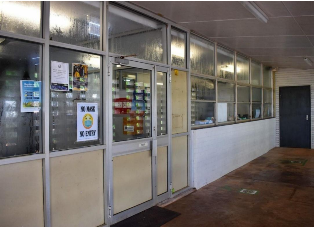
3 Miwatj Health's Yirrkala clinic is struggling with lack of space and urgently needed repairs
