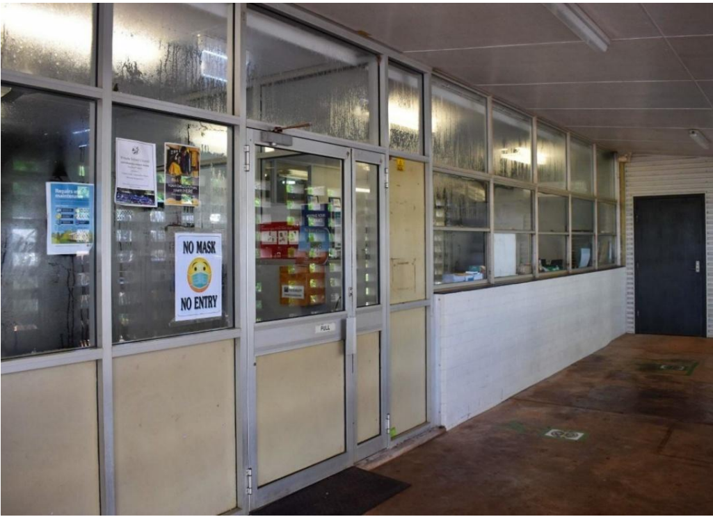
3 Miwatj Health's Yirrkala clinic is struggling with lack of space and urgently needed repairs
